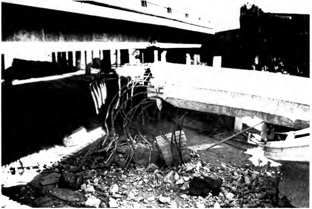
Photo 13. Column of overcrossing at the Golden State Freeway and Foothill Freeway interchange [4].
